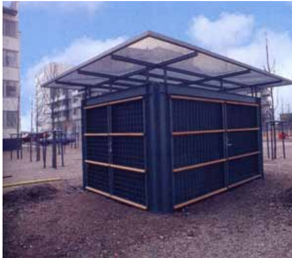
Transformatorstation (Norra hamnen Helsingborg)
