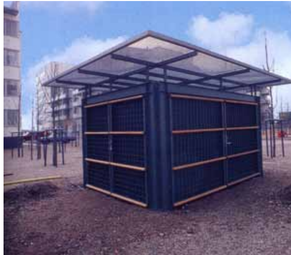
Transformatorstation (Norra hamnen Helsingborg)
